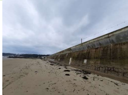
Wave return wall to mitigate strength of wave attack.
